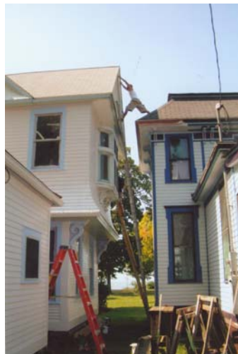
Frank Isherwood's second cottage, at left. Even the side gable towers above the neighbor. The actual main roofline is even higher. Note how easy (!) it is for my stepson to walk from roof to roof. The gap between the Isherwood cottage and the house on its other side is even LESS!
